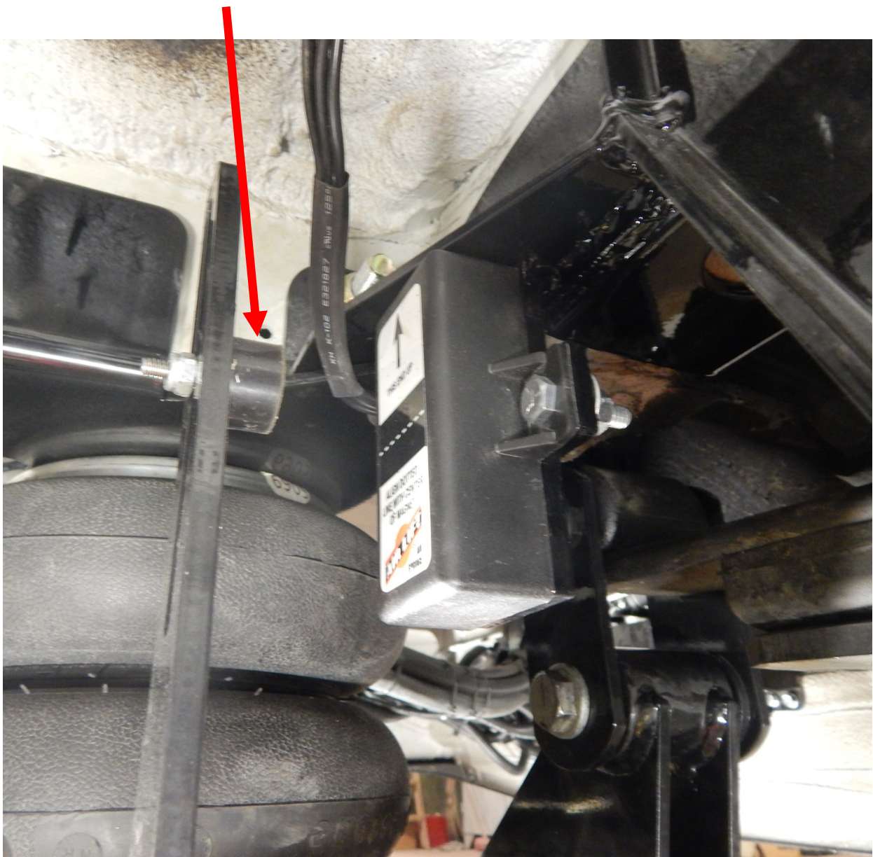
Magnet in operating position
