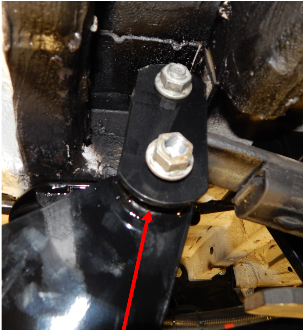
Spacer on the link goes on the bottom towards the poly bushing in the swing arm
