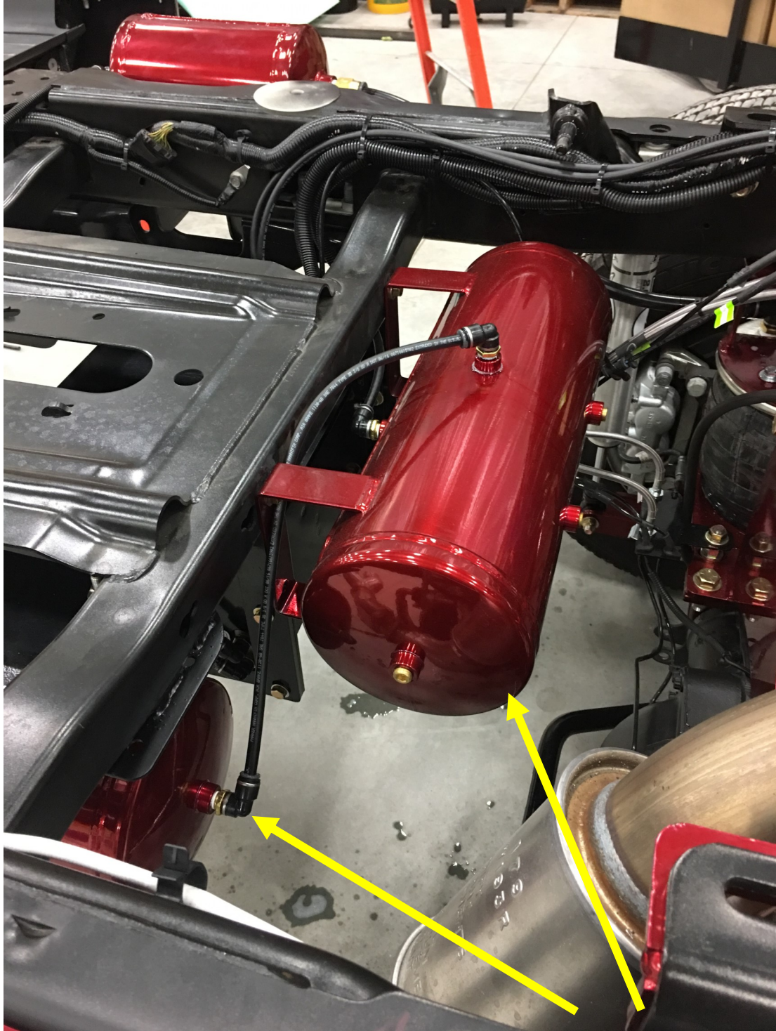
Air tanks plumbed together
