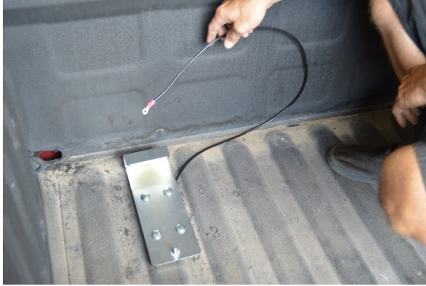
(Fig. 8) Driver's side Mounting Bracket installed. Note the ground wire attached to front inside bolt. The other end attaches to the Electronic Level Sensor on the tank.
