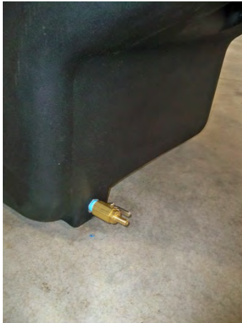
(Fig. 8) Ball valve installed
