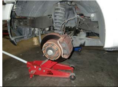
Hold up the beam with a floor jack while the vehicle frame is supported.
