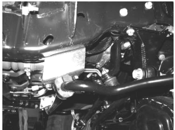
View of outer driver side frame rail
